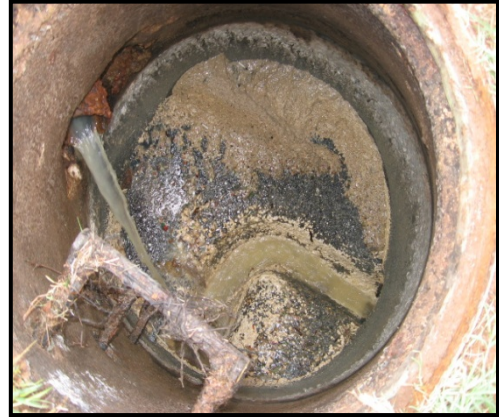
Figure 1. CMU Sewer grease blockage, 2008
